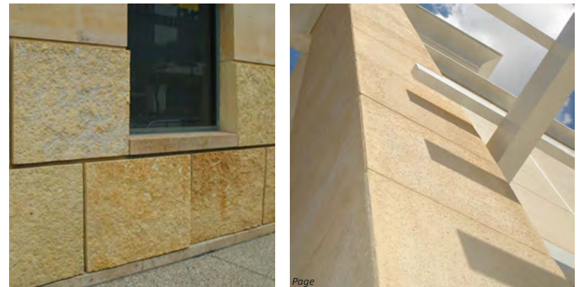
Use of natural stone enhances building color and texture (above left and right).
